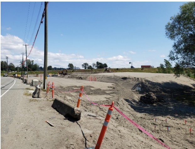
S1: River Road West Roundabout – Preload/embankment fill placement for watermain construction. Taken July 10, 2020
