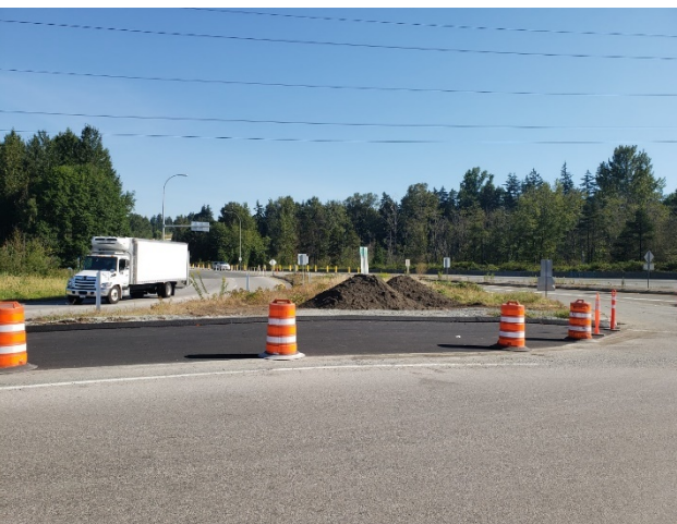
S4: E01 Detour – Recently paved left turn lanes from Nordel Way EB to Hwy 91 NB/Alex Fraser Bridge. Taken July 27, 2020
