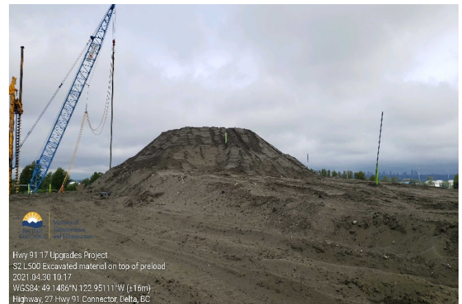
S2: Weigh Scale Rd west side excavated material on top of preload. Taken April 30, 2021
