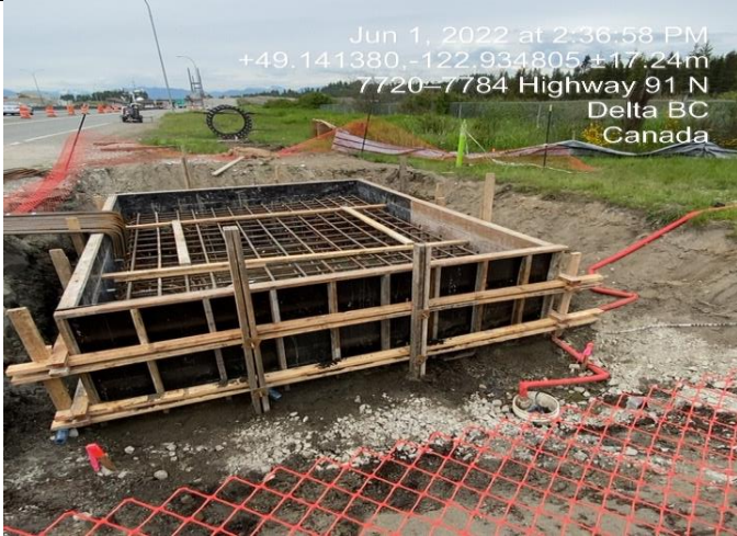
Photo 71: L2400 (G). Formwork for a guide sign that will be poured with concrete.
