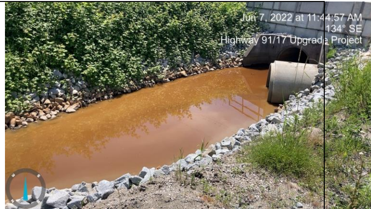
Photo 82: Low water levels and elevated turbidity at Silda culvert discharge location.
