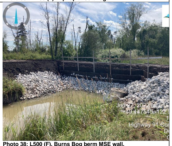
Photo 38: L500 (F). Burns Bog berm MSE wall.
