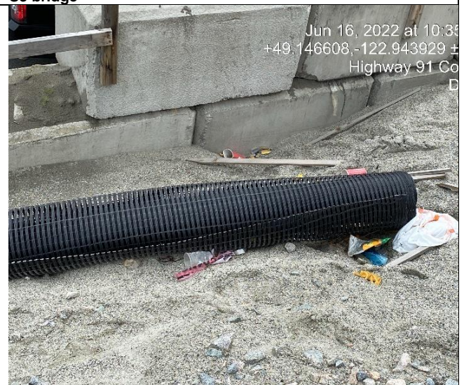
Photo 32: L1150 (F). S3 bridge littering
