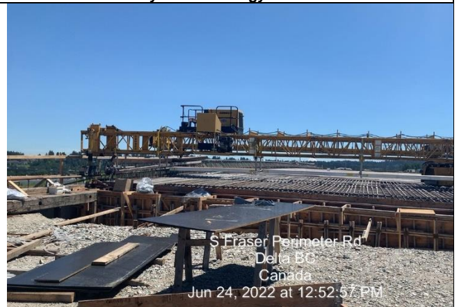
Photo 92: JBs S3 Bridge worksite cleanup – Haz Mat and general construction waste removed from work area.
