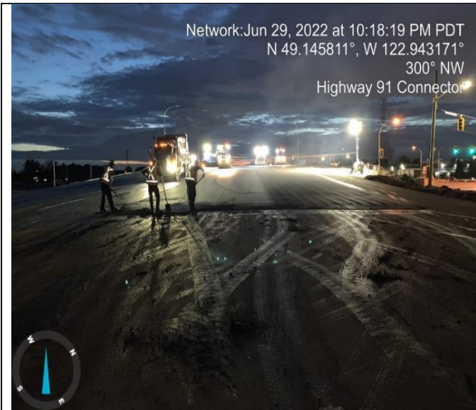
Photo 93: L500, S3 bridge ramp. All Roads paving the top lift on the S3 bridge ramp.
