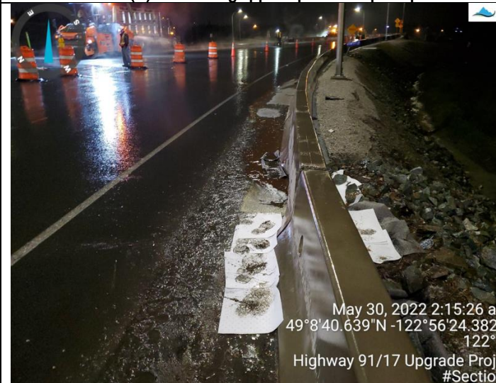
Photo 55: L600 (I). Tack spill.
