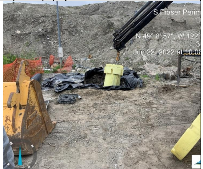
Photo 90: Hazardous waste material from Sunbury Mounds removed from site by Secure Energy.
