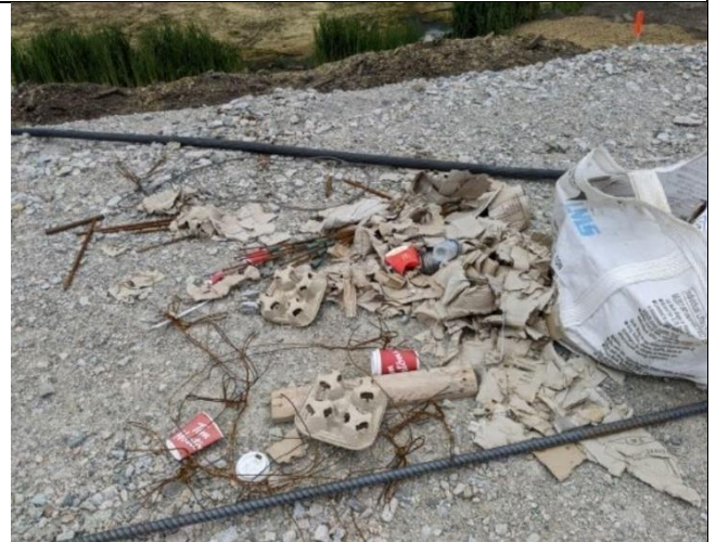
Photo 84: S3 Bridge - Waste and food garbage observed without appropriate containment/disposal.
