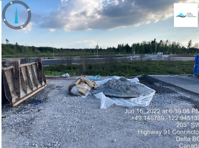
Photo 85: S3 Bridge - waste concrete left on site, inadequate containment.
