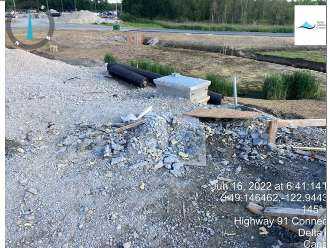
Photo 86: S2 Bridge - waste concrete and garbage not disposed of properly.
