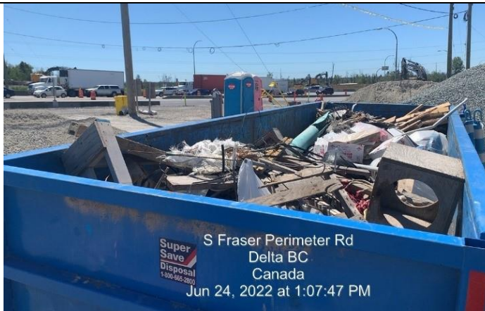
Photo 91: Jacob Brothers S2 Bridge worksite cleanup – general waste sorted into appropriate receptacle.
