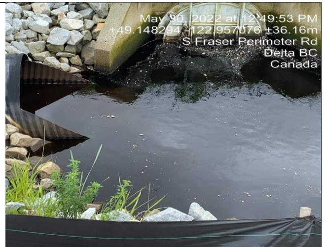
Photo 76: L525. Resolution of elevated turbidity at 96 St Ditch US.
