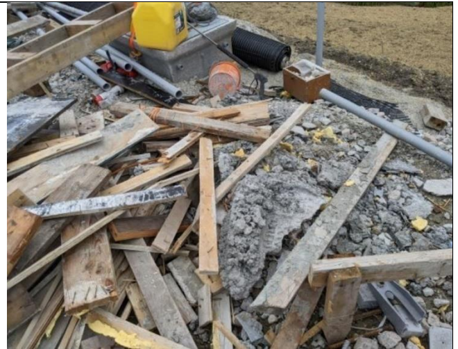
Photo 88: S3 Bridge – jerry can with diesel fuel without secondary containment. Waste concrete and garbage not disposed of properly.
