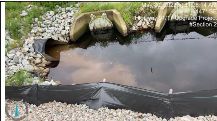
Photo 75: L525. Unauthorized pumping to 96 St Ditch US.
