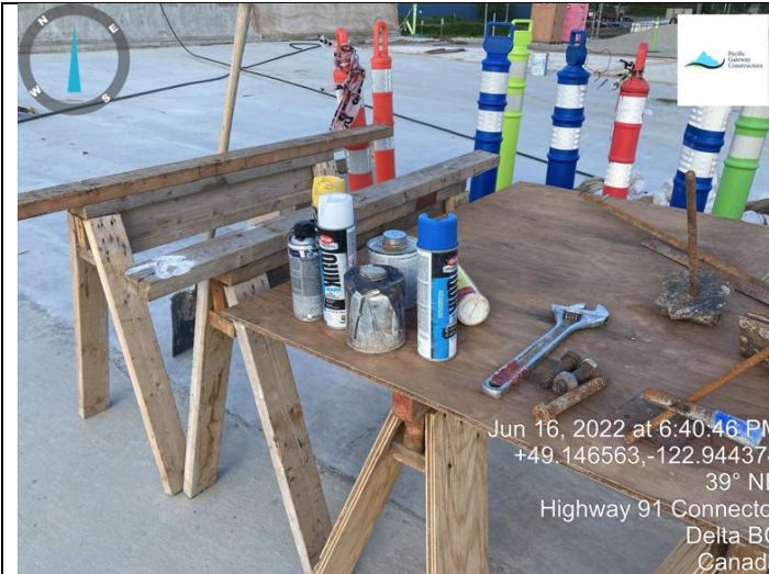
Photo 87: S2 Bridge – hazardous materials without secondary containment.
