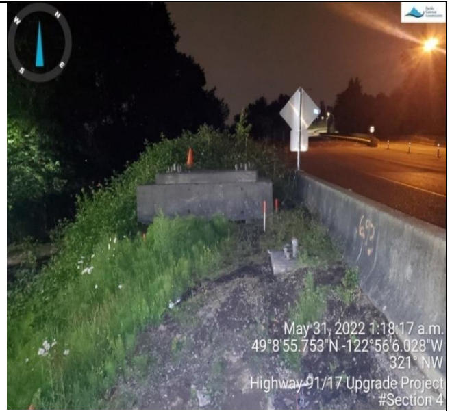
Photo 70: L600 (G). Removed streetlight.
