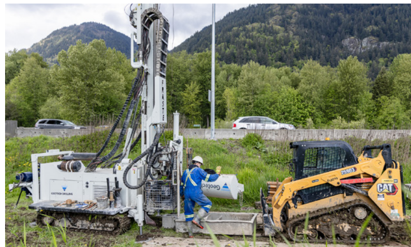
Field investigations are underway along Highway 1 to understand soil conditions between Abbotsford and Chilliwack to help plan for future construction.
