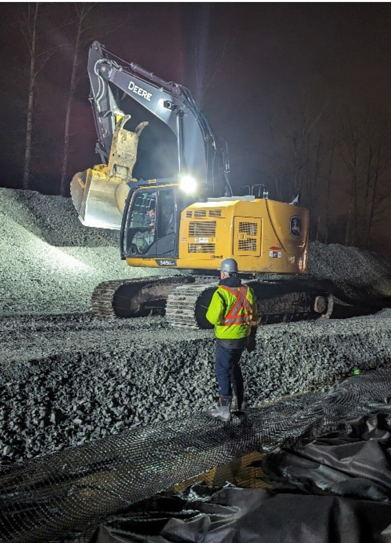
Nighttime work is ongoing to lessen impact on traffic during peak travel times. Visit drivebc.ca for the most up-to-date information.
