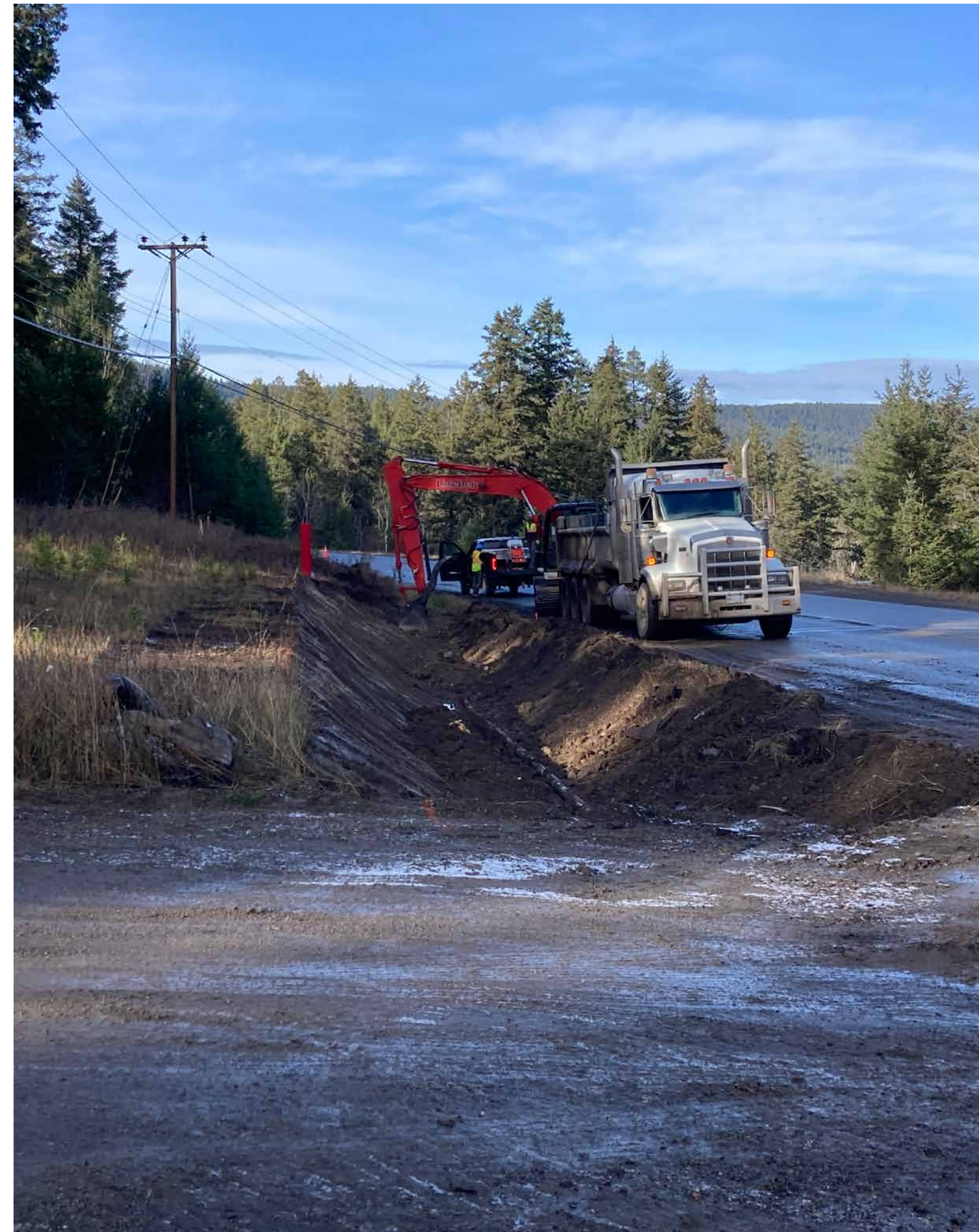
Phase 1 ditching work was completed last fall in the Hodgson Slide area.
