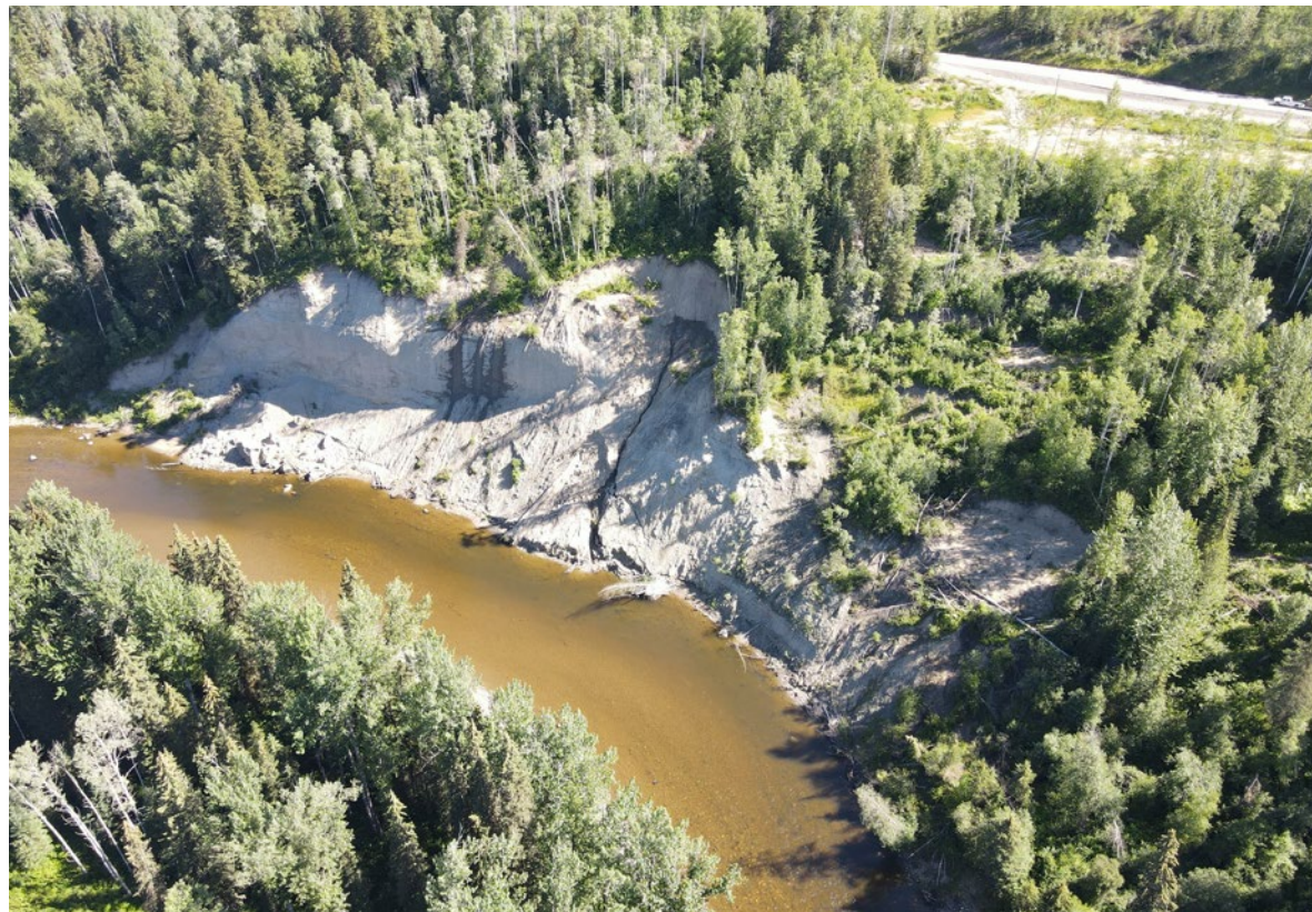
Photo of the embankment to be stabilized along the Cottonwood River.
