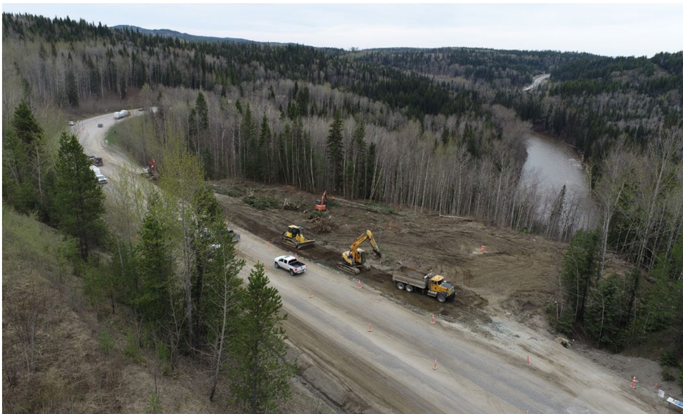
Photo of crest unloading work along Highway 97 at Cottonwood Hill adjacent to the Cottonwood River.
