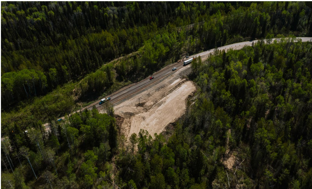
An aerial view of the Highway 97 at Cottonwood Hill Project, where weight was removed from the top of the slide adjacent to the highway.
