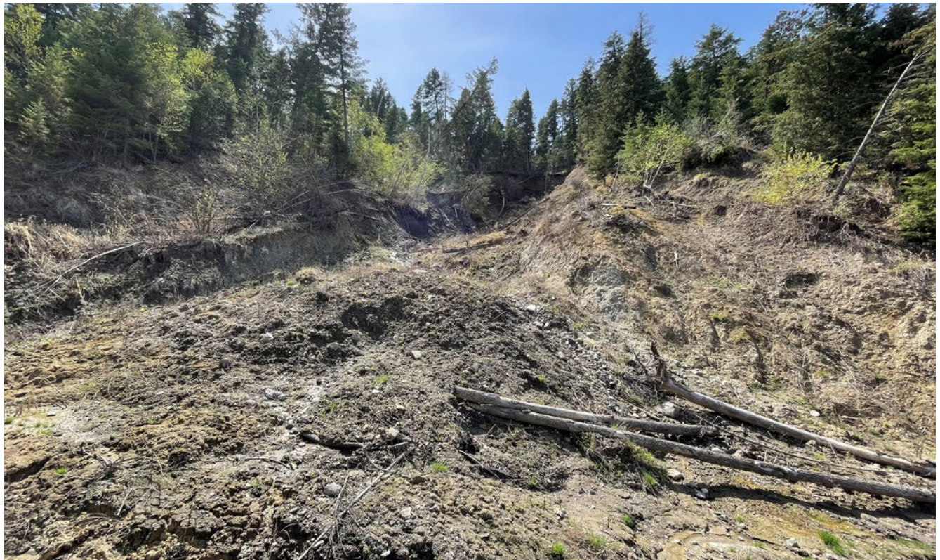
Photo taken from Dog Creek Road, at the bottom of the Dog Creek Slide.
