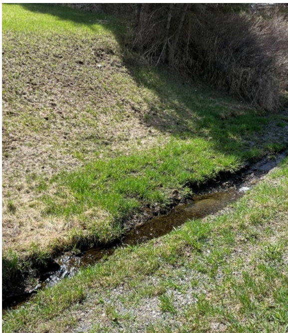
Phase 1 work includes the clearing and widening of ditches within the Hodgson Slide area.
