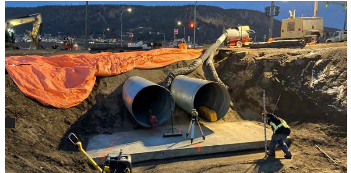
Crews installing culverts as part of the surface water management on the Highway 20 at Hodgson/Dog Creek Road.
