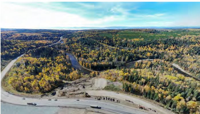
Aerial view of construction crews working to stabilize the slope alongside the affected section of Highway 97 at Cottonwood Hill.
