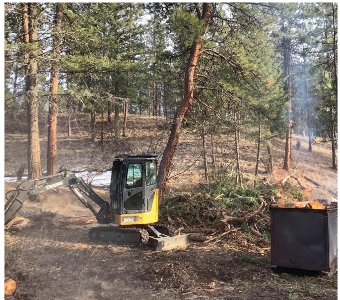
Figure 26. Burn box for debris management to limit site disturbance during a fuel management project in Ellison Provincial Park.
