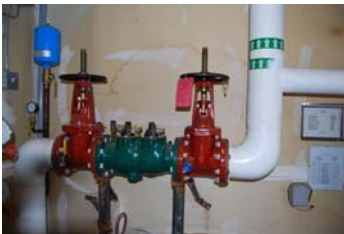
Installed in conformance with the BC Building Code
