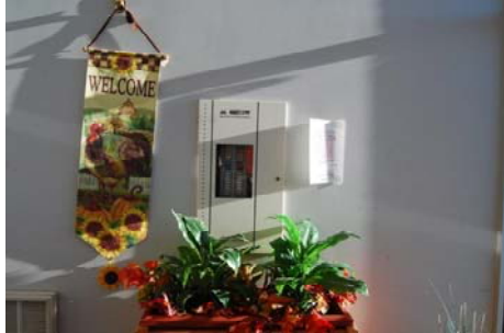
Inspections – Interior (Fire Alarm Control Panel)
