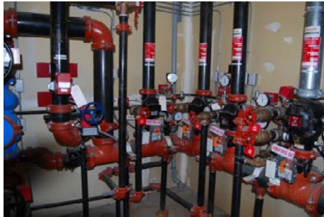
Sprinkler Room – Interior
