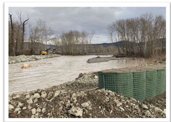
Coldwater River – temporary flood mitigation structures – Spring 2022
