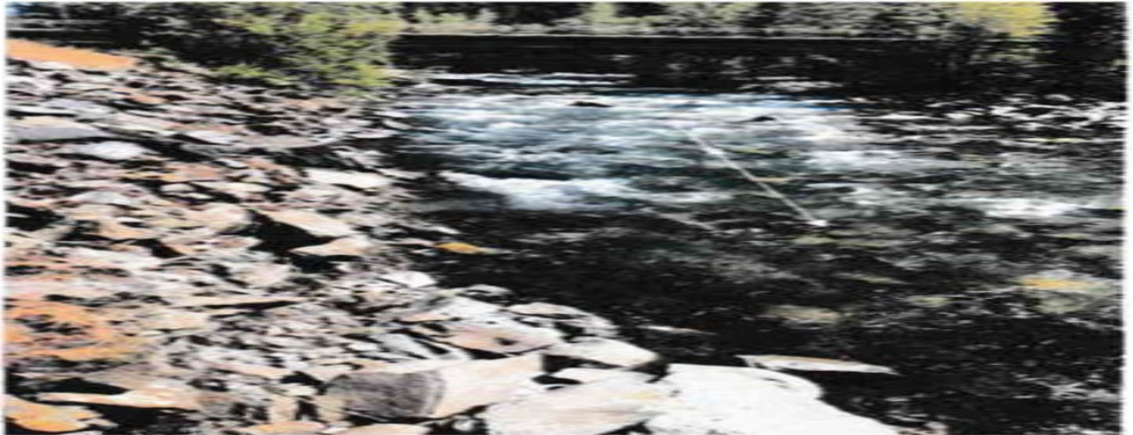
Figure 5: Site 4 Riprap Lost August 25, 2020
