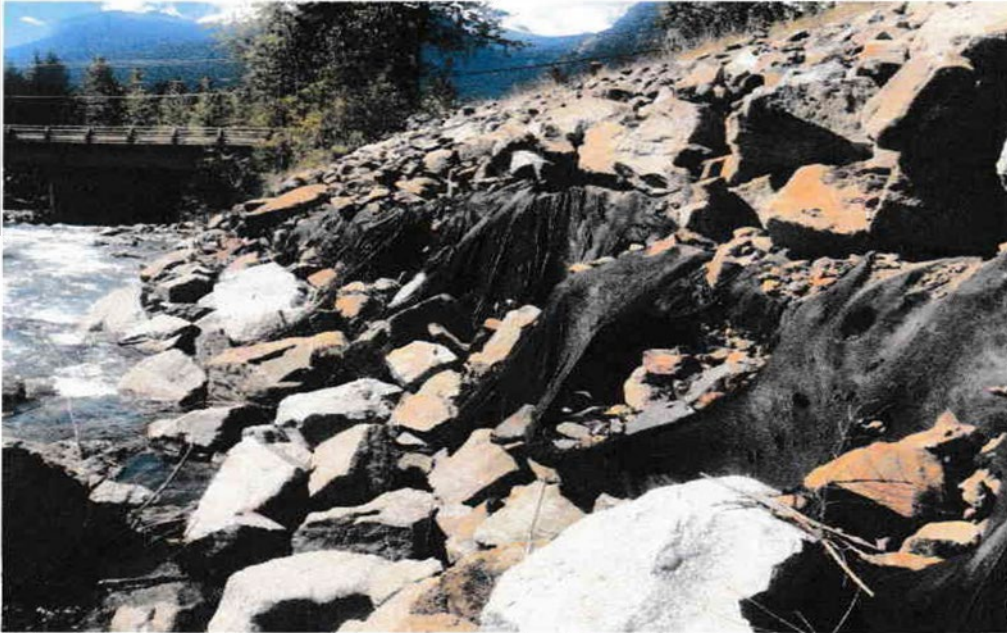
Figure 7: Site 5 Dike Erosion August 24, 2020
