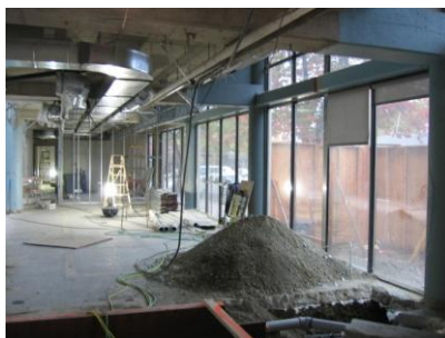
Extensive renovations were needed to convert the former pre-trial centre to the community court
