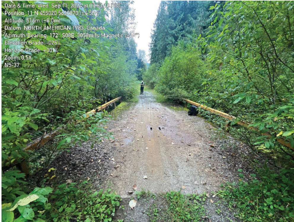
Overview of Bridge N5-037. Note the cut holes in the deck for machine lift.
