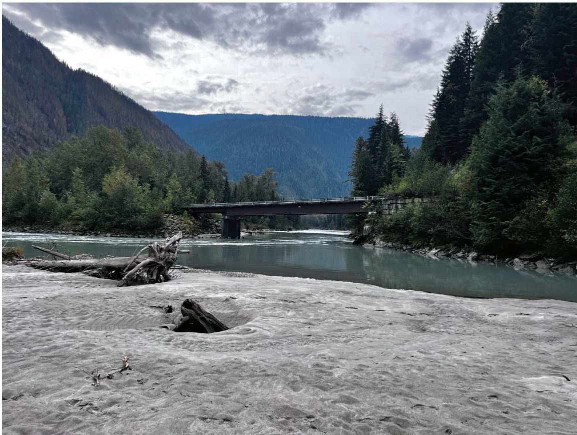
Bridge N5-035. Looking downstream. Bush side lock block wall visible on the right.
