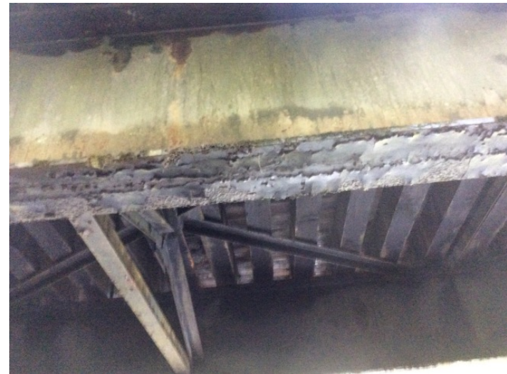
surface corrosion on bottom of girder flange
