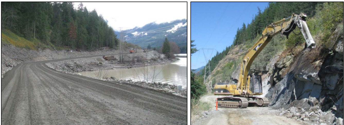
Figure 10. Recent capital projects raised previously flooded roadbed near KM 24 (left) and widened narrow sections of roadway (right). (Source: FSR overview presented at in-SHUCK-ch PIEVC workshop, Squamish, B.C.).
