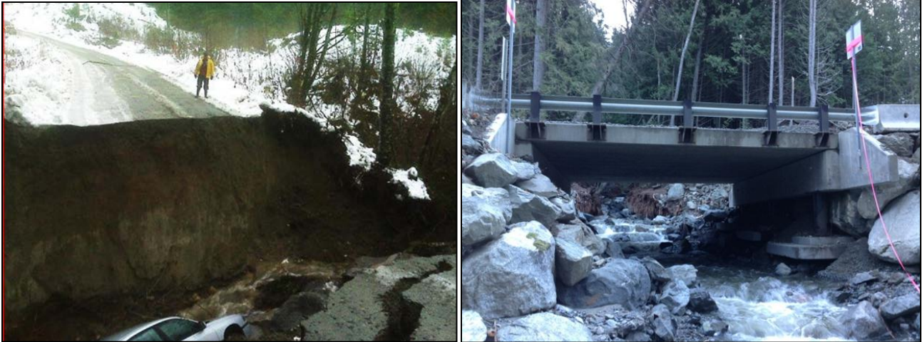
Figure 7. Large culvert washout (left) and bridge abutment undercutting (right) caused by high stream flows. (Source: FSR overview presented at in-SHUCK-ch PIEVC workshop, Squamish, B.C.).
