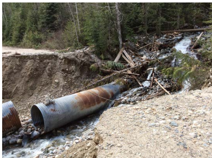
Figure 5. Culvert washout at KM 17 following storm damage in September 2015. Photo courtesy of Daryll Cairns.
