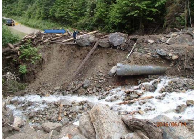
Figure 6. Culvert washout at KM 17.3 following storm damage in September 2015. Photo courtesy of Daryll Cairns.
