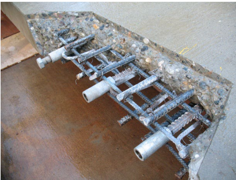
Figure 5: Properly saw cut repair area free of weak, loose or damaged concrete. Surfaces are clean and ready for formwork. The full diameter of the rebar has been exposed, and all areas have been cleaned to remove all traces of loose concrete, dirt, debris and rust.
