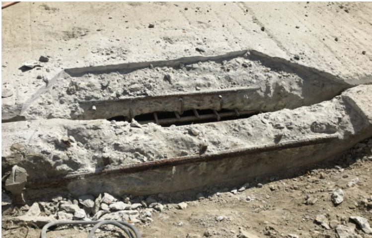
Figure 2: Site preparation for a repair is in progress. Repairs have been initiated by saw cutting a perimeter area around the repair area. This example depicts a “deck beside ballast wall” configuration of precast bridge components which is no longer used for new FSR bridges.
