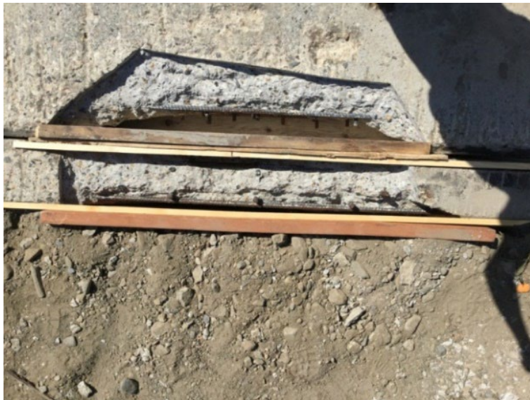
Figure 9: Formwork placed after removal of damaged concrete and prior to placing CIP mixture for ballast wall and deck panel repair.
