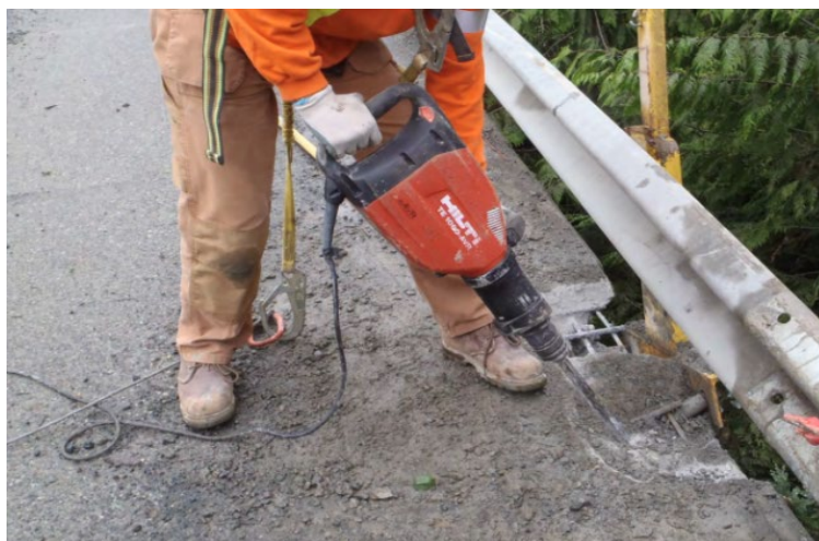
Figure 3: Mechanical removal of damaged concrete near a guardrail post at the edge of a bridge with a chipping hammer.
