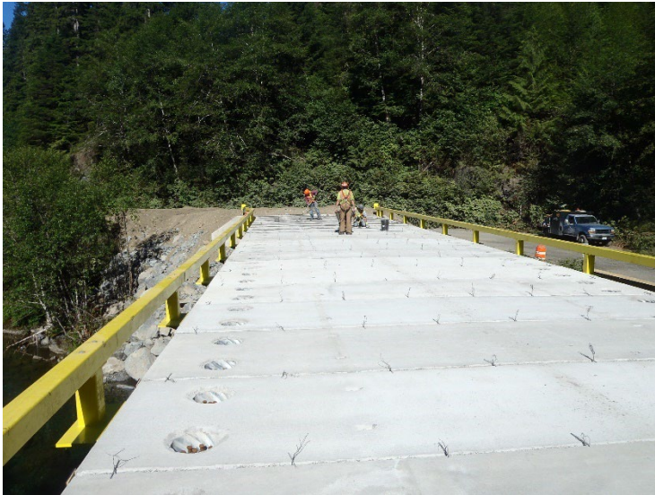
Figure 1: Bridge crew starting to place CIP mixtures for the superstructure of a new two lane steel girder composite concrete deck bridge a) in transverse deck panel joints, and b) in shear-stud blockouts for deck to girder connections.
