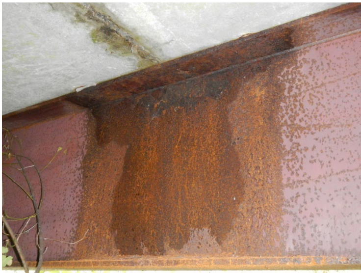
Figure 10: A leaking transverse deck panel CIP joint causing corrosion of a steel bridge girder. Poor Quality Control of surface preparation, mixing, placement and/or curing can be detrimental to FSR bridge durability and longevity.
