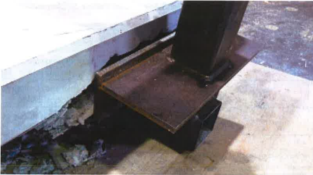
Figure 2 Typical Observed Failure of the Modified HSS Guide Retrofit Rail
