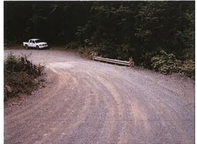
Poor horizontal and vertical alignment and increased bridge width
