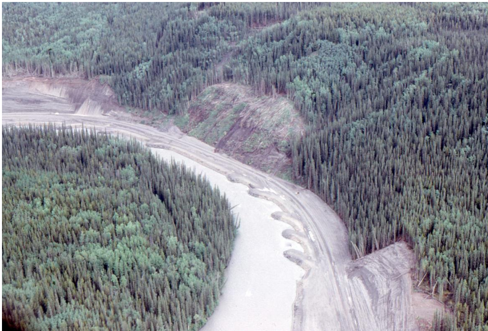
Photo 15. September 1974 photograph of the rail grade under construction. The photo shows the rail grade being constructed in the active channel of the Klappan River.
