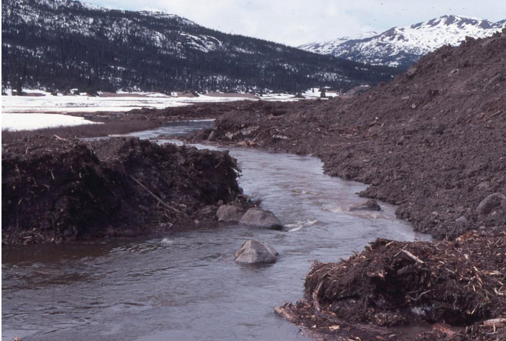
Photo 16. A photo of rail grade construction effects along the Spatsizi headwaters near the Skeena divide. The photo shows material wasted directly into the river. Photo date is June 1976.
