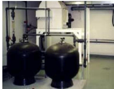
Sand filters and microfilter
