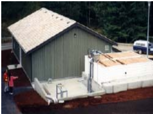
Influent pump tank, bioreactors and Process Building
