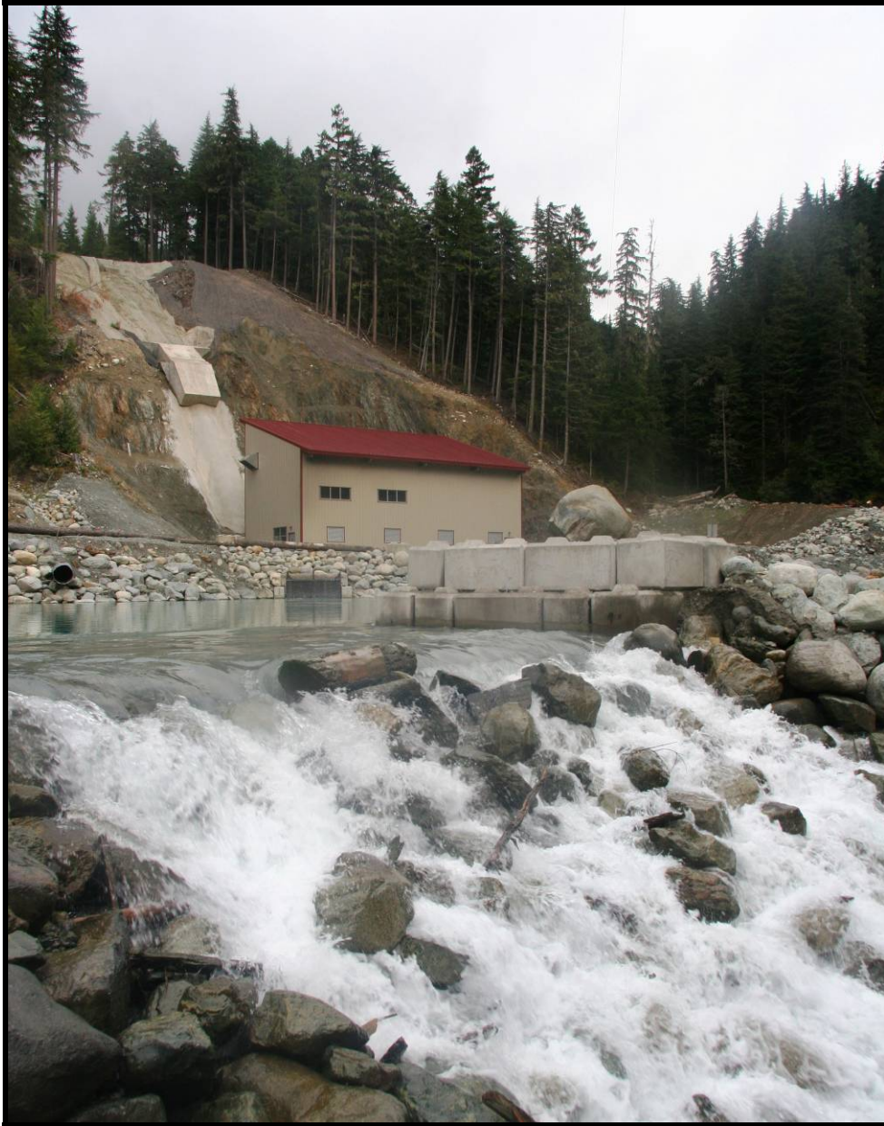
Fitzsimmons Creek IPP Powerhouse and Snowmaking Intake Pond
