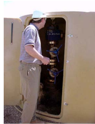
CO 2 injector within injector housing Source: Petroleum Technology Research Centre
