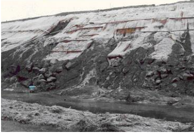
Failure of erosion-control matting.
