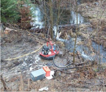
Streamside water supply pump - the pump and motor are seated in a containment tray and the ground is buffered by a tire.
