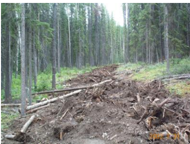
Reclaiming a road. Soil has been loosened and large debris and root balls pulled over the roughened surface.
