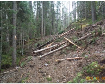
Recontoured trail on a steep slope. The site is to be seeded with grass to control erosion.
