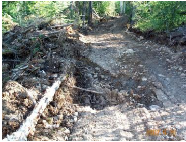
Trail washout caused by improper drainage and organic debris in the sub-grade.
