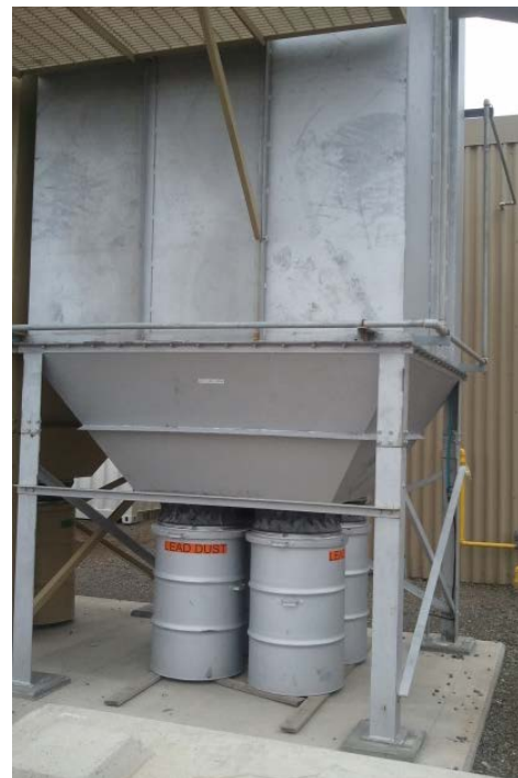
Figure 5: Lead dust collection barrels of an exhaust filtration system.
