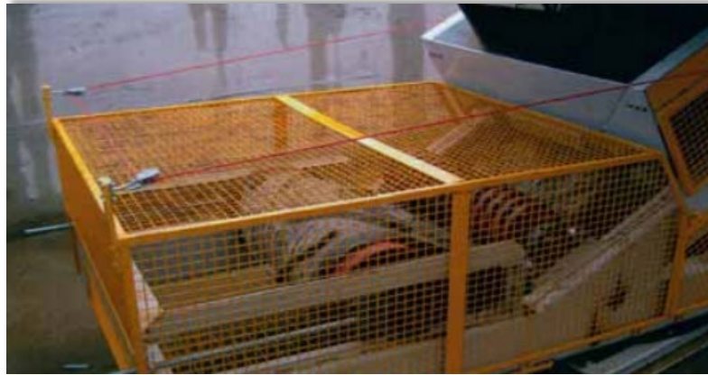
FIGURE 2:EXAMPLE OF A GUARD PROTECTING THE TAIL PULLEY OF A CONVEYOR
