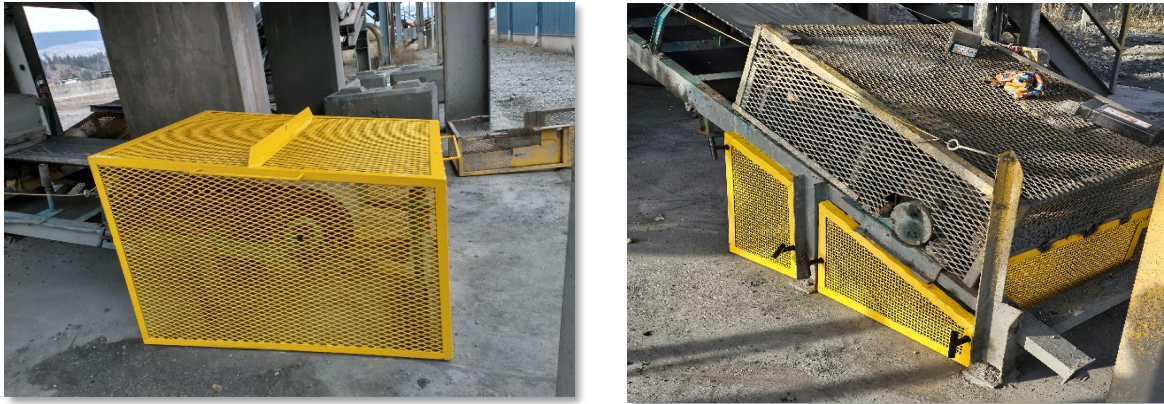
FIGURE 5: EXAMPLE OF GUARD PROTECTING TAIL PULLEY
