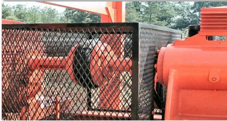
FIGURE 1:EXAMPLE OF A GUARD AROUND A MOTOR DRIVE COUPLING
