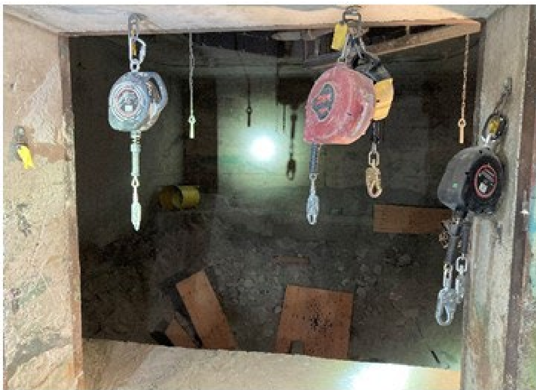
FIGURE 1. Surge Bin Door with Collapsed Materials.
