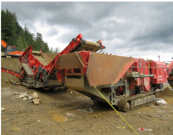
FIGURE 1. Rock Crusher with Feeder Conveyor
