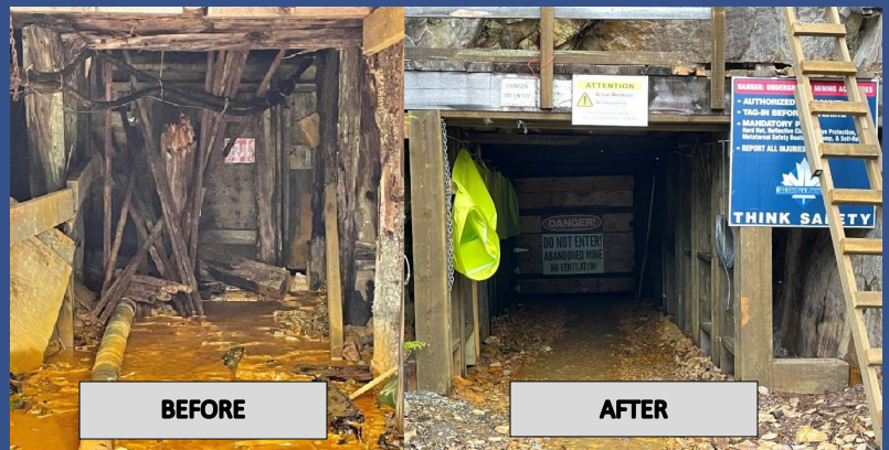
View of 5400 Level entrance before and after replacement of the timber support, showing the new door and new timber throughout the portal. This work enabled safe access to the 5400 Level entry.
