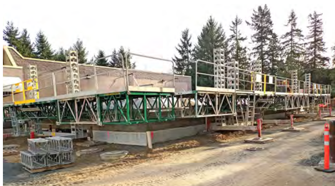
Figure 4. Hydraulic scaffolding used for rapid installation of bricks to build up the core walls of the new freezer/cooler.
