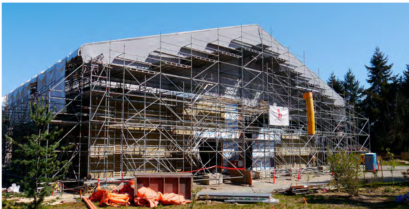
Figure 6. Current stage of construction (May 2024), with wooden shake siding to be installed over all old and new freezer/cooler exterior walls, and a new roof to be installed over the entire facility (50,000 ft 2 or 4,645 m 2 ) in tandem with this expansion project.
