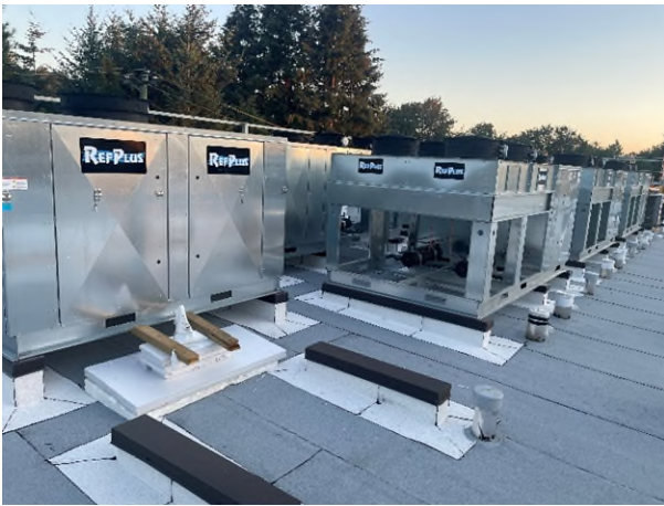
Figure 2: Enclosed scroll type compressors on the roof.
