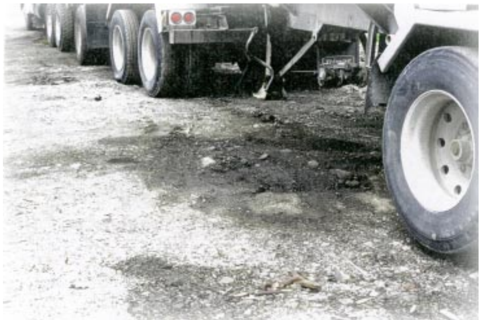
Visible hydrocarbon stains in marshalling yard
