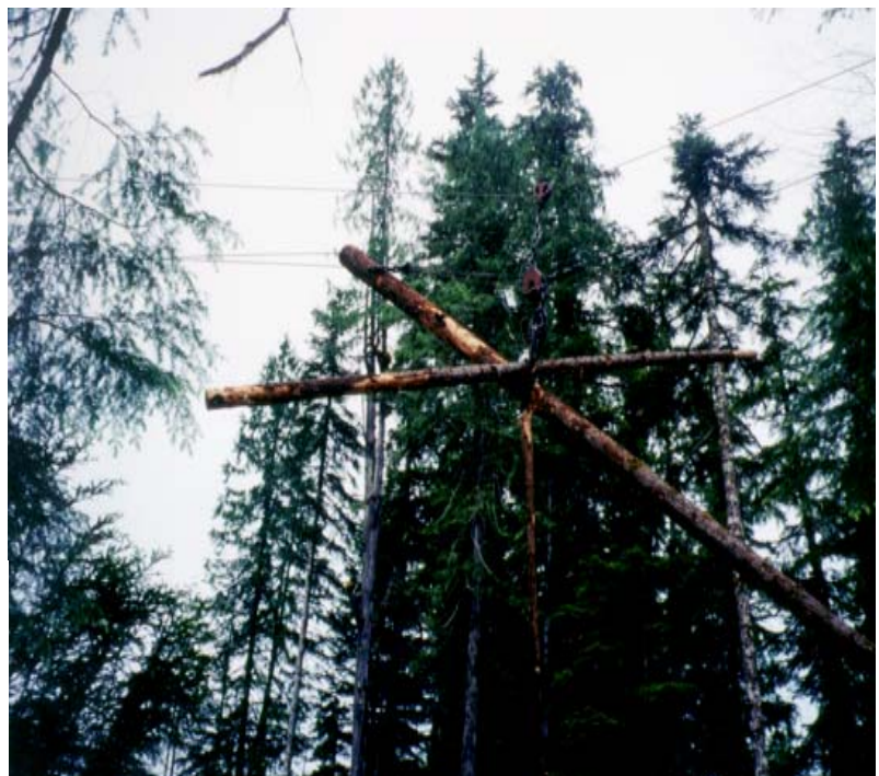
In the Gold River Forest Operation in Block E520 full-suspension logging was undertaken through a Riparian Reserve Zone during the permitted fisheries window using a yarding corridor and full stream protection .
