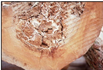
Brown crumbly rot decay with white mycelium.
