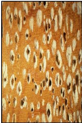
Advanced stage of decay caused by H. abietis .
