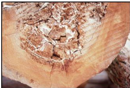
Brown crumbly rot decay with white mycelium.
