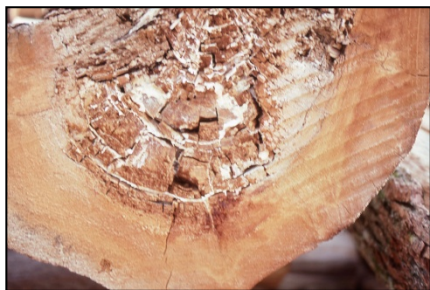
Brown crumbly rot decay with white mycelium.
