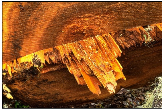
Decay caused by C. rivulosa in western red cedar.
