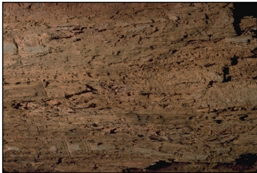
Advanced decay caused by F. officinalis in western larch.
