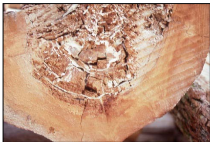
Brown crumbly rot decay with white mycelium.
