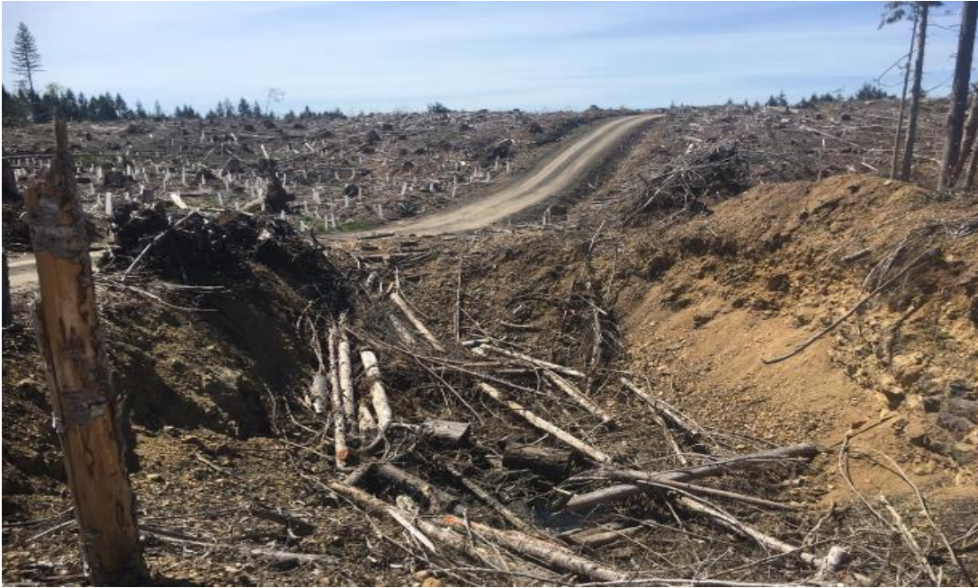
Figure 50. This spur road slopes down towards the wetland and is hydrologically connected (wetland is on either side of the road at the bottom of the hill). The amount of bare erodible soil will include the length and width of this bare ground, multiplied by the fraction of fines (< 2 mm) and the fraction considered to be hydrologically connected.
