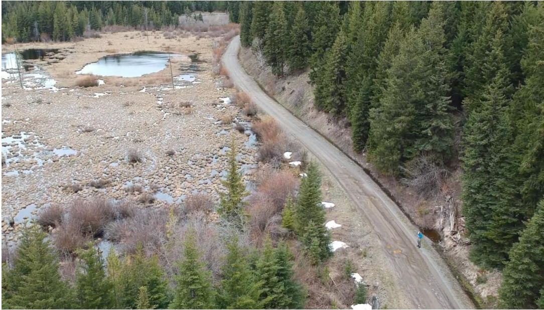
Figure 24. Ditch on the right of the road carries water from an unmapped seasonal stream over 300 m in the ditch, passing several blocked culverts, before passing under the road, through a still functioning culvert, and into the wetland (on left of road). Water no longer follows a natural water course.
