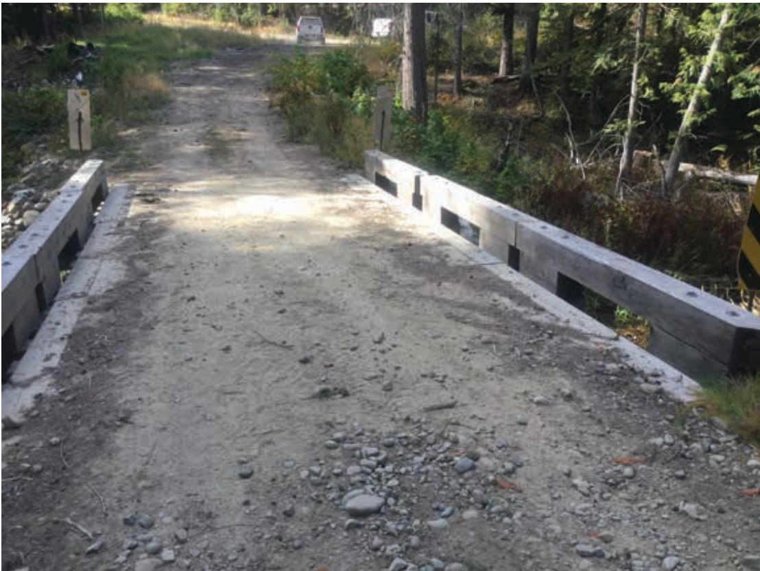
Sediment accumulation on bridge deck over a fish bearing stream
