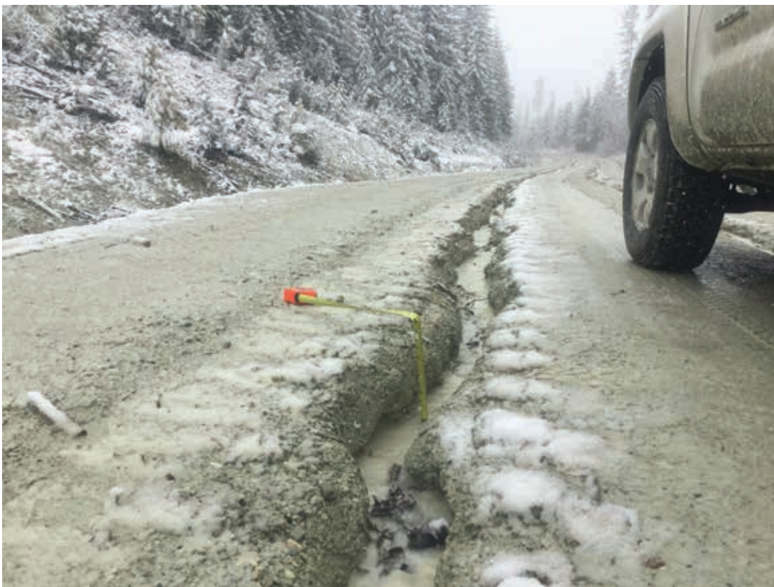
Road ruts channeling water and eroding the road surface.
