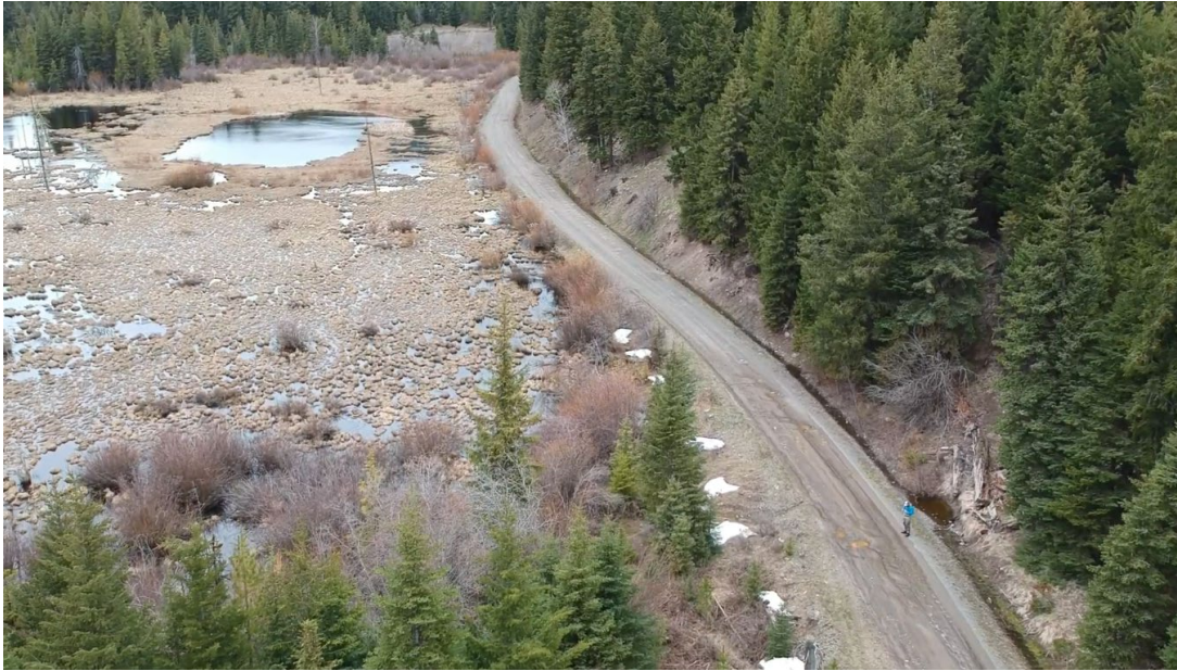
Figure 24. Ditch on the right of the road carries water from an unmapped seasonal stream over 300 m in the ditch, passing several blocked culverts, before passing under the road, through a still functioning culvert, and into the wetland (on left of road). Water no longer follows a natural water course.
