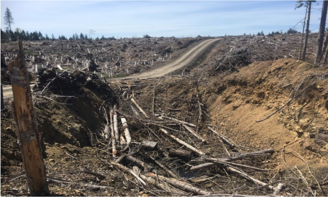
Figure 50. This spur road slopes down towards the wetland and is hydrologically connected (wetland is on either side of the road at the bottom of the hill). The amount of bare erodible soil will include the length and width of this bare ground, multiplied by the fraction of fines (< 2 mm) and the fraction considered to be hydrologically connected.
