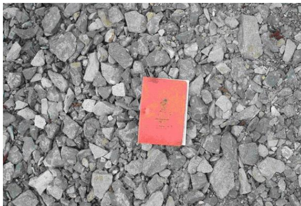
Photo 3. The road surface on the slope draining toward the stream crossing (Section 1) was all free draining crushed rock. Overall average bare erodible ground exposure was at most 1%.
