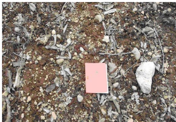
Photo 4. Bare erodible ground made up 70% of the surface of the ditches in Sections 4 and 5. These sections were also fully connected to the stream.
