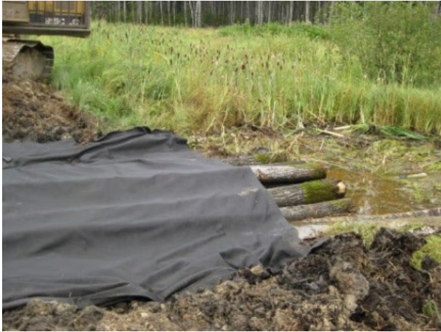
Photo #1: Log bundle built two or more logs high with a separation layer placed over the top to prevent the voids from becoming filled with road surfacing material. The bundle was used to allow low volume flow through a road in a wetland. Note the logs extend past the edge of fill to allow water to easily enter or exit the structure.
