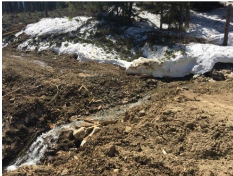
Photo #4: Example of a log bundle location within a NCD showing that the structure was removed before snow melt and before flows increased; log bundles are most appropriate for predominantly dry channels with periodic seepage or low flow.
