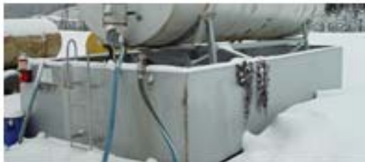
Tank in a box
