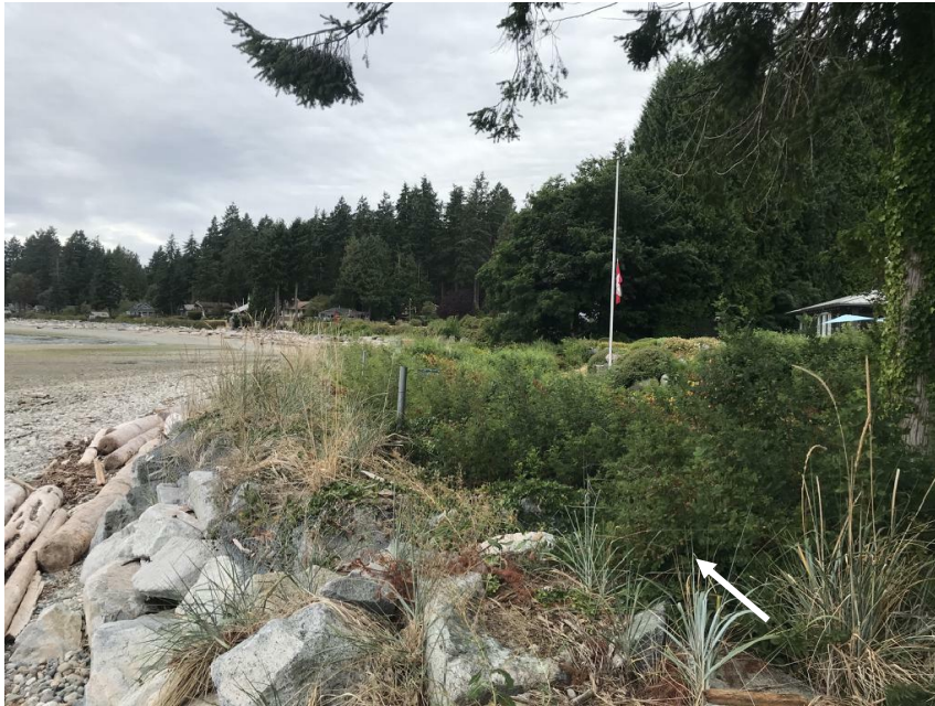
FIGURE 6.13 View westward and down Stephens Creek along the oceanfront. White arrow shows flow direction. Note the left bank of the creek is armoured with riprap. Placemark 114, August 6, 2021.
