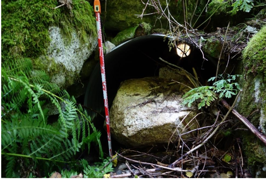
FIGURE 9.2 View of boulder blocking 800 mm diameter culvert along Roberts Creek tributary 12.2 in the upper eastern portion of Roberts Creek (latitude: 49.470°, longitude: -123.579°). Photo DSC09534, August 25, 2020.
