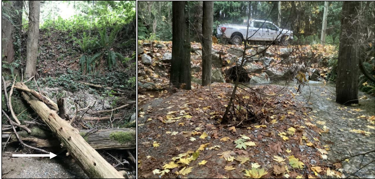
FIGURE 6.14 View downstream of the culvert inlet at the Lower Road crossing of Stephens Creek. The left image shows conditions at the culvert inlet on August 6, 2021. The white arrow shows the location of the culvert invert obscured by wood debris. The right image shows conditions at the same location in November 9, 2023 approximately two years after the crossing was washed out and replaced (photo courtesy of Pierre Aubin of BCTS). Note the higher elevation of the culvert and streambed on the right image.
