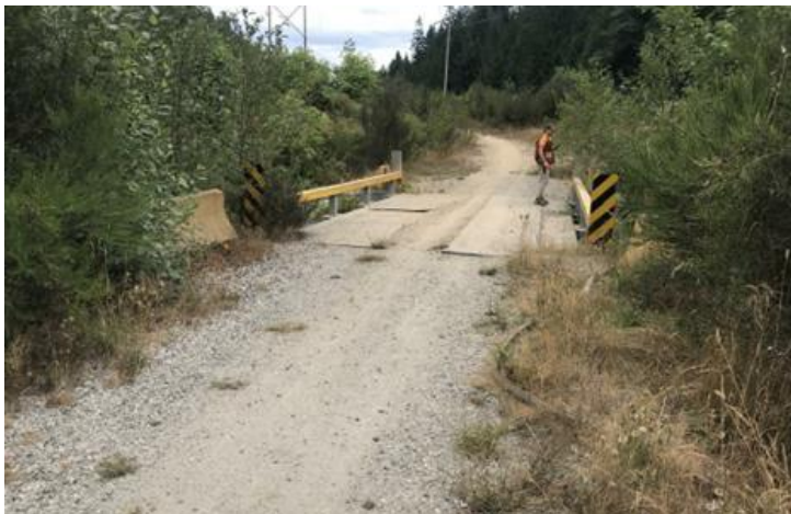
FIGURE 4.1 View westward along the BC Hydro ROW. Bridge crosses Stephens Creek at an elevation of approximately 161 m. Photo DSC09916, August 6, 2021.
