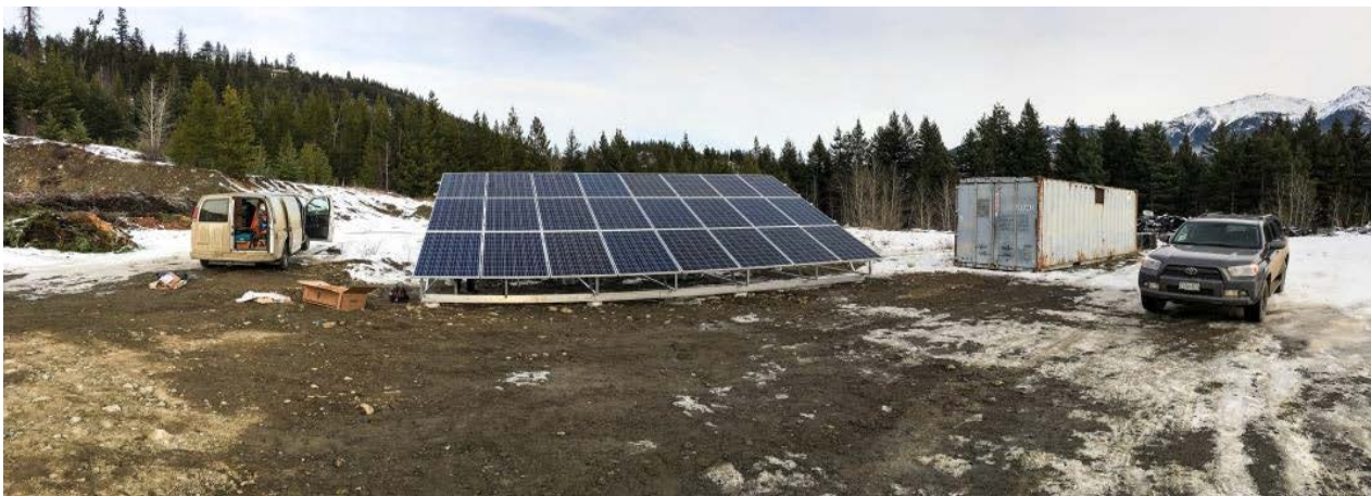
Solar array at Transfer Station
