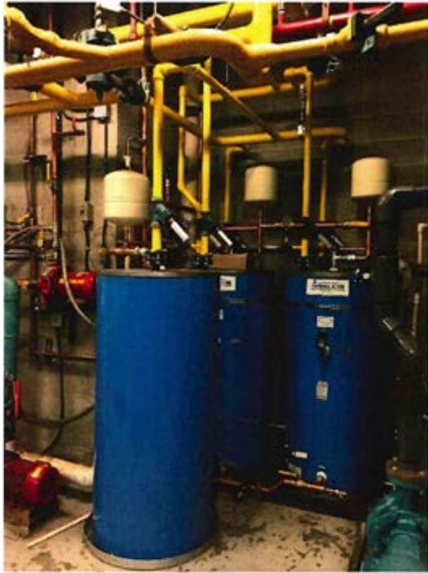
Hot Water Heat Recovery Tanks
