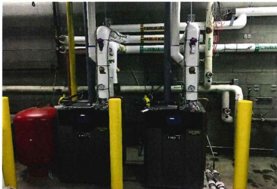
New Condensing Boiler
