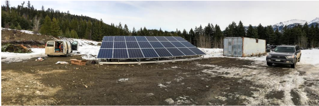
Solar array at Transfer Station
